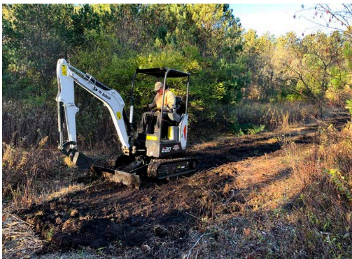
Volunteer Bob Richardson uses the Friends' new mini excavator to construct ski trail at Willow River State Park.
